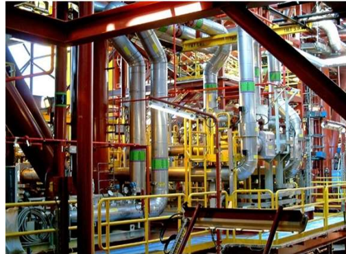
Keeping the pipes clean is vital for our health
